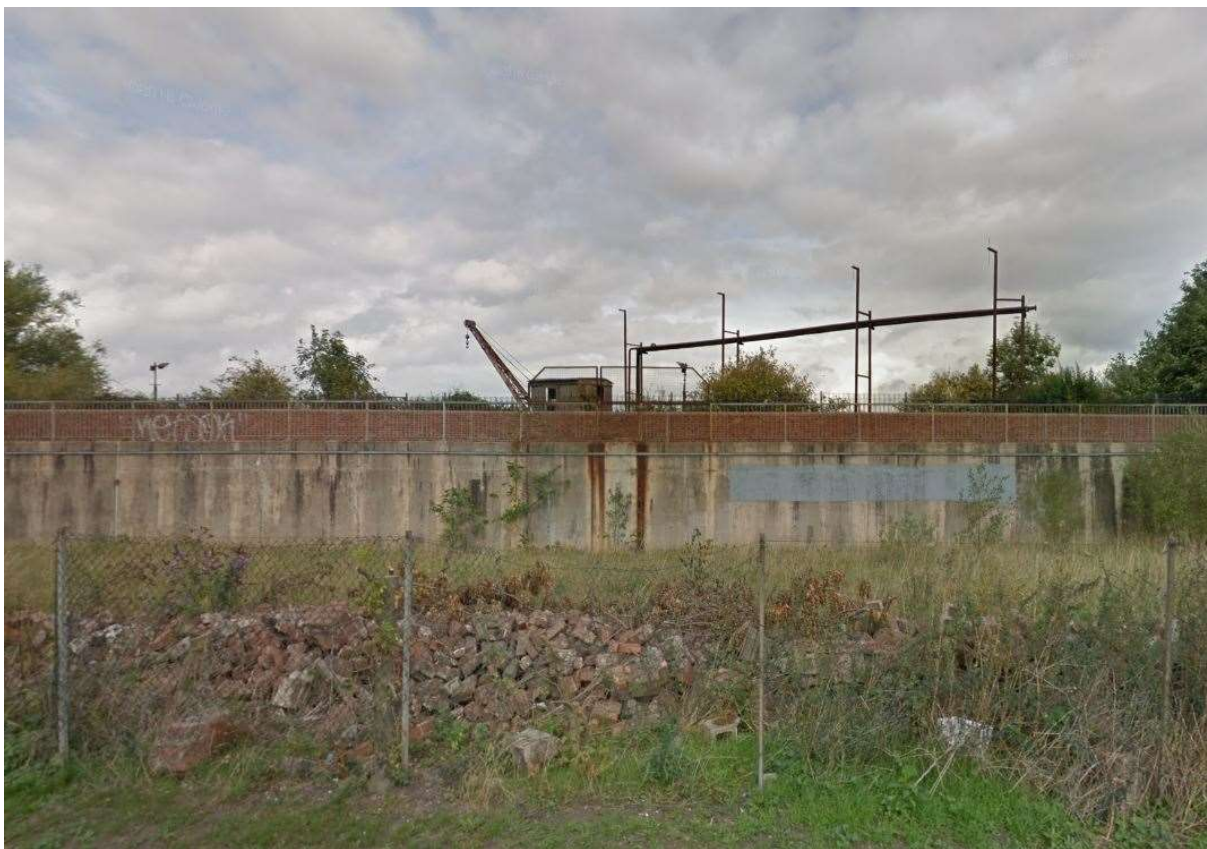
Figure 4 - View from the A19 showing site constraints in the form of 2No. flood defence walls
